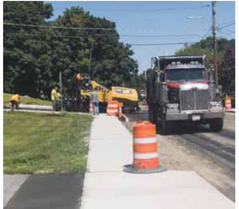
The Norwood DPW is already deep into spring projects, including repaving of many streets and continued pipe relining.
